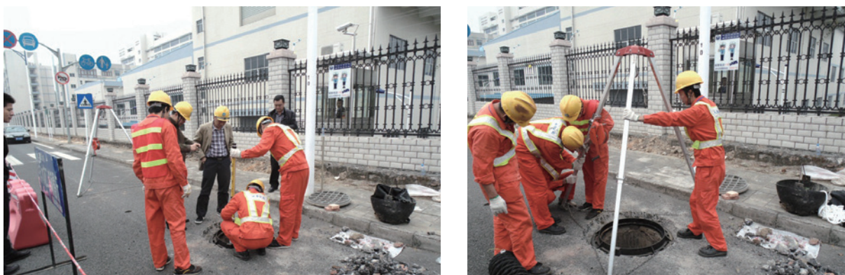
Maintenance of drainage pipelines by Shenzhen Grand Industrial Zone Water Co., Ltd.
