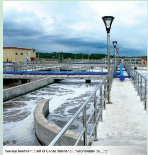
Sewage treatment plant of Gaoan Xincheng Environmental Co., Ltd.
