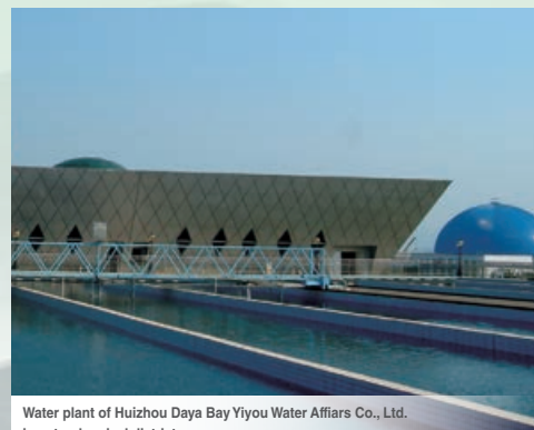
Water plant of Huizhou Daya Bay Yiyou Water Affairs Co., Ltd. in petrochemical district
