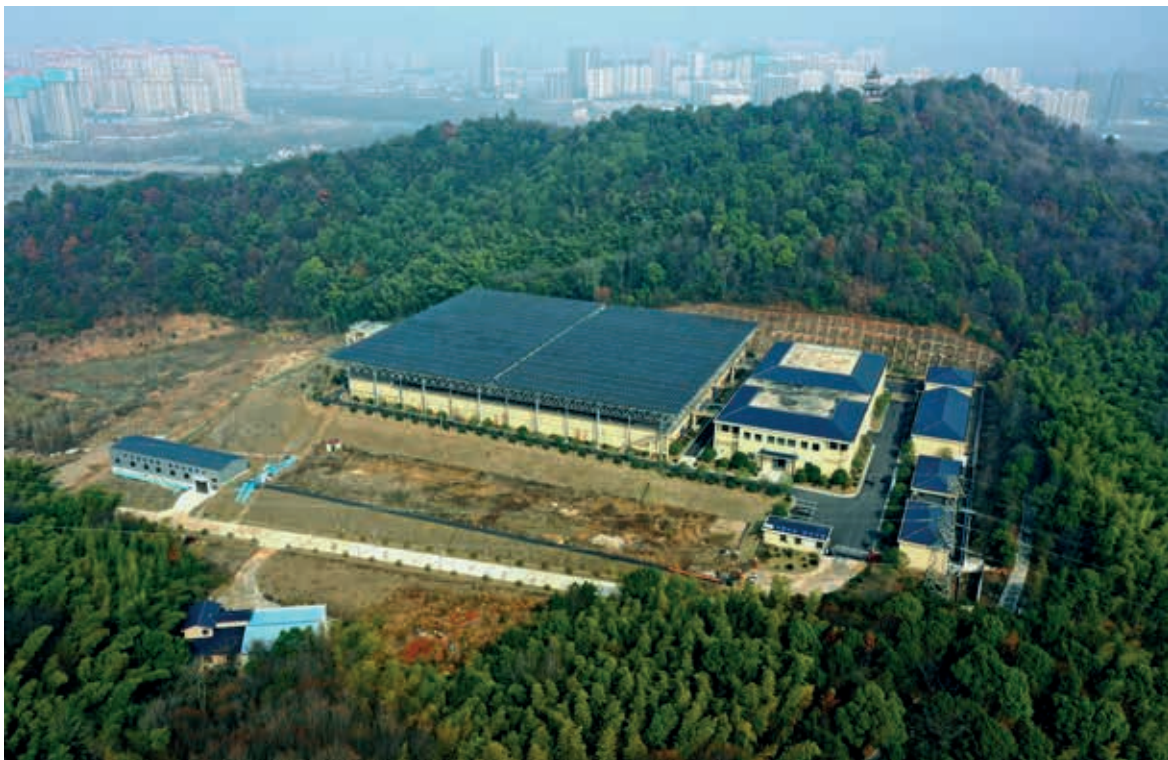
PV equipment installed at Nantaihu Water Plant, Ningxiang on top of the reaction pool and the horizontal-flow sedimentation pond
