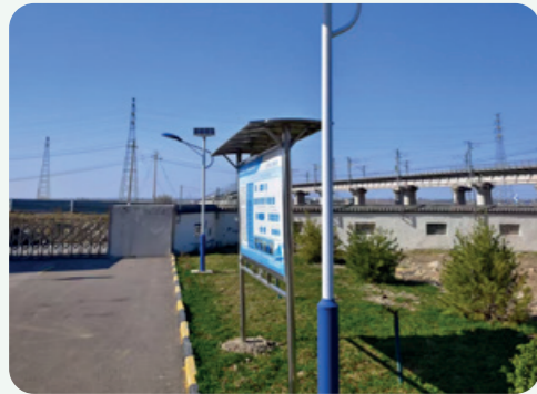
Upgrade energy-efficient lighting in the plant area
