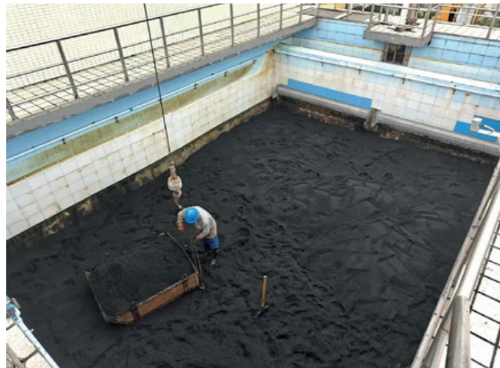
Chongqing Qiaoli Water Affairs Co., Ltd. adopted a non-stop operation method to thoroughly clean the filter material and filter heads of the filter pools
